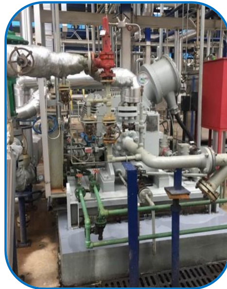
▲ CNOOC Huayue Chemical Company P3001A/B Hydrogenation Charging Pump GSB-Q4-25/1100 Power: 185KW
